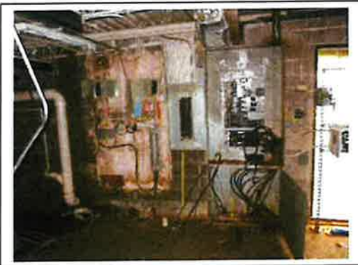
Building Interior Electrical Panels
